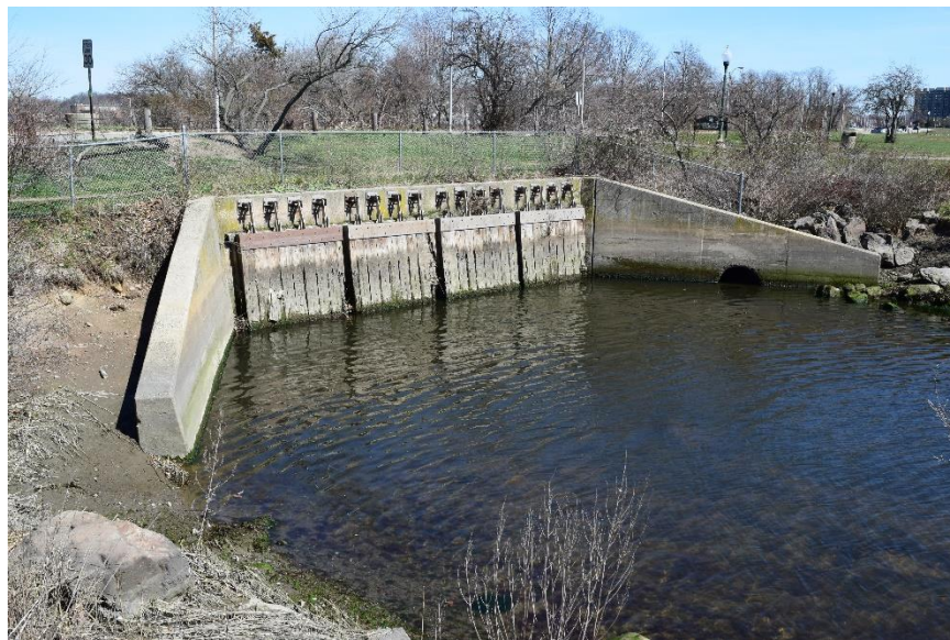
Photo 2-21: Wooden tidegates at Captain Thomas Blvd. at the mouth of the Cove River.
