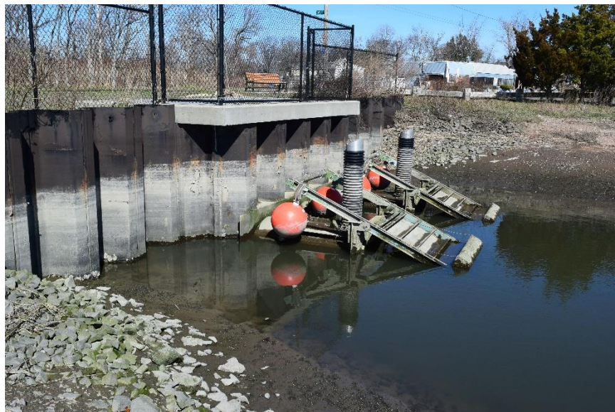
Photo 2-17: Self-regulating tidegates at Beach Street
